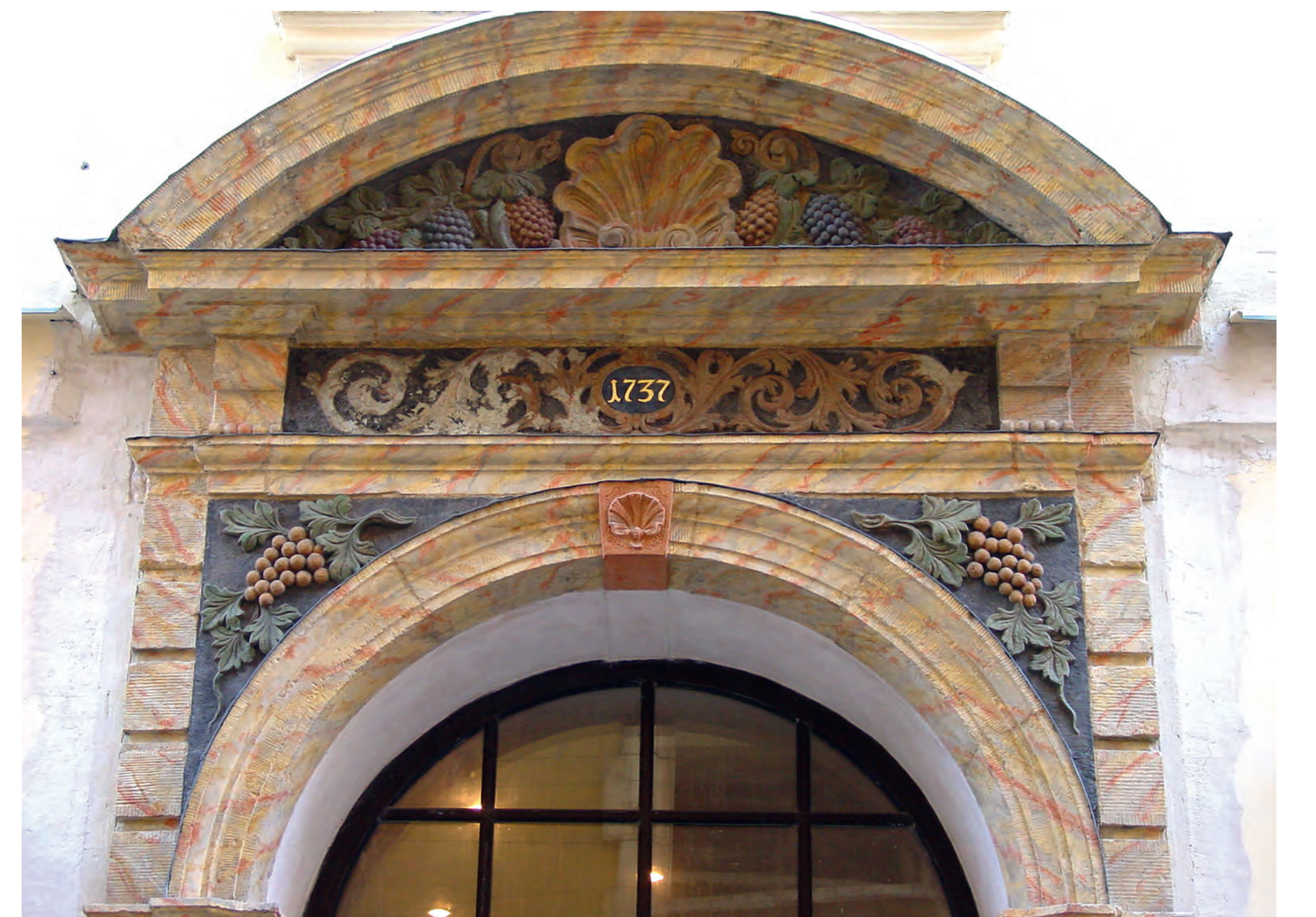
6. Portal in Riga, Kramu str.3, gypsum mortar between the stone blocks during construction, 1737.
